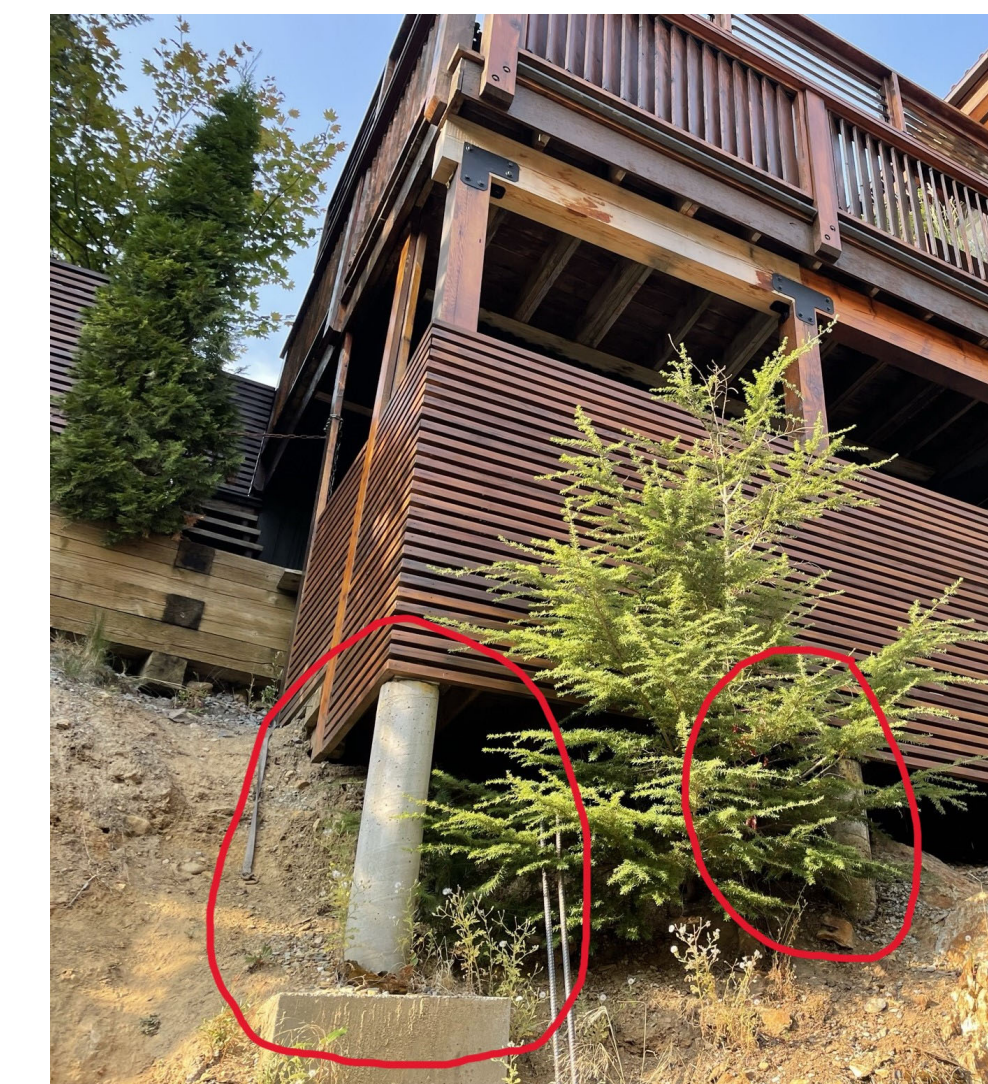
IMAGE OF ENCRDACHING POSTS
