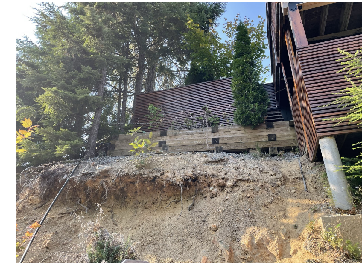
IMAGE OF ENCRDACHING POST & SLOPE
