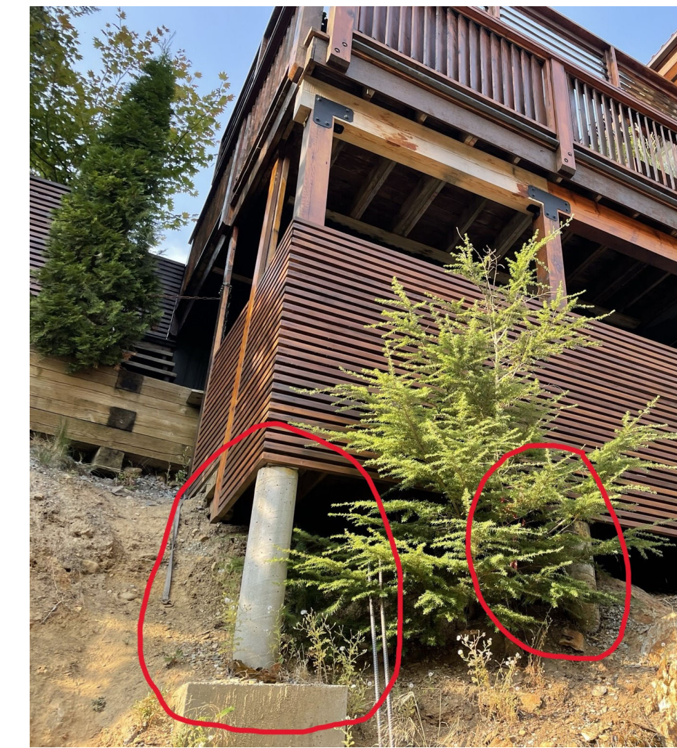
IMAGE OF ENCRDACHING POSTS
